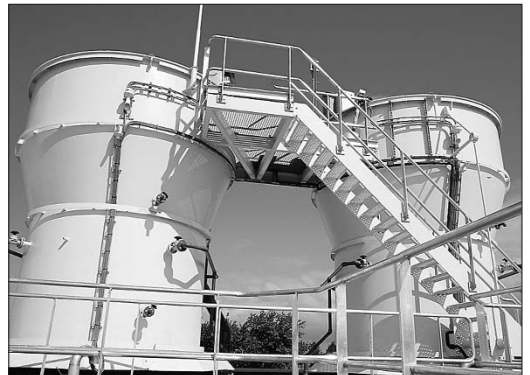
The full-scale calcium phosphate recovery installation at Geestmerambacht sewage works, The Netherlands, was visited by Conference participants.
