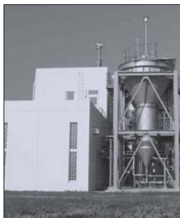
Commerically operational full-scale struvite recovery installation at Shimane Prefecture sewage works. Photo : Unitika Ltd, Japan.
